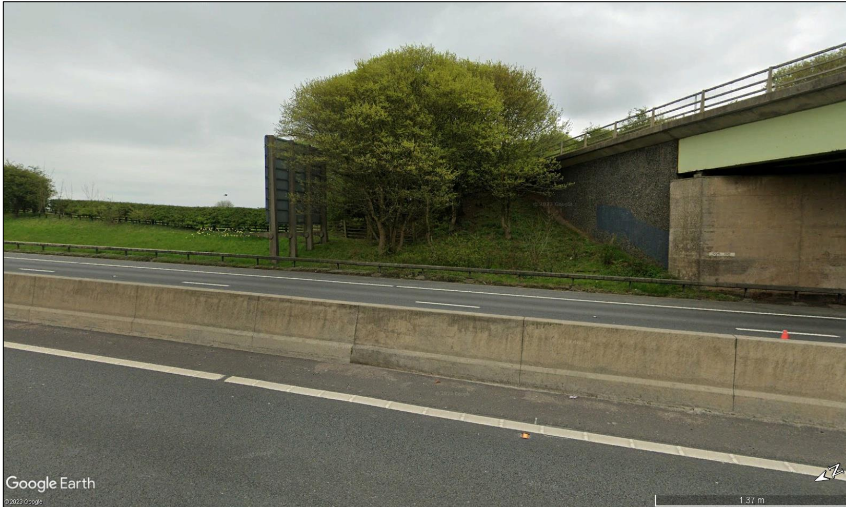
View towards reflecting panels from road receptor 7 (representative of the extent of screening for road section 6-7)
